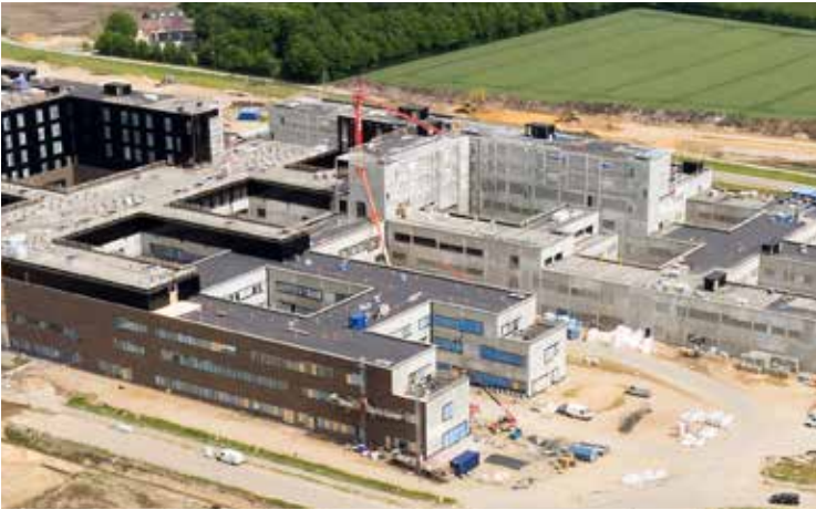
Hospital Godstrup, Denmark
